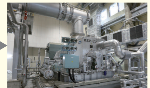
蒸気タービン発電設備 Steam-turbine power-generating equipment
